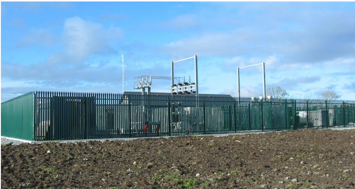
Figure 2-9 Typical Substation Compound
